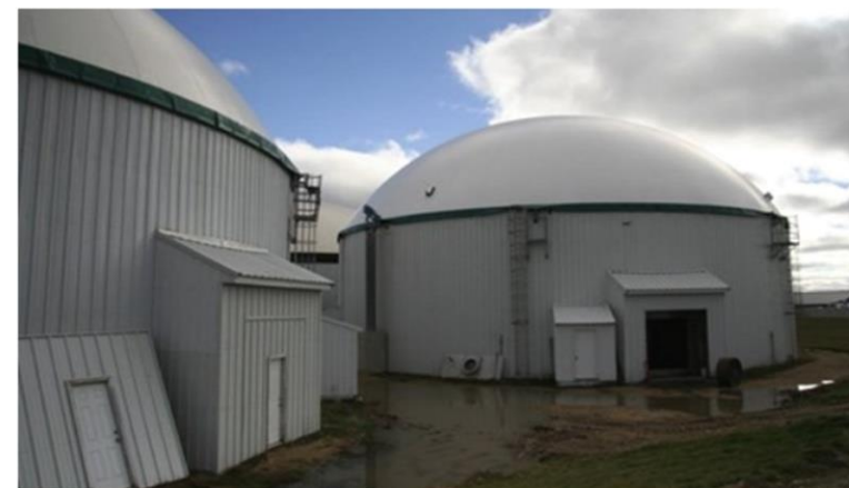
Clean Fuel Partners installed a new roof on digester tank #2 in November 2015. Photo Credit: Clean Fuel Partners
