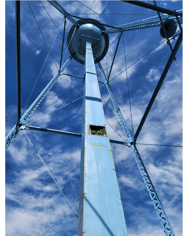
Water tower with leaking riser pipe
